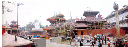
View of temples in Kathmandu Darbar Square with restoration ongoing at Kal Bhairav shrine and Jagannath temples
